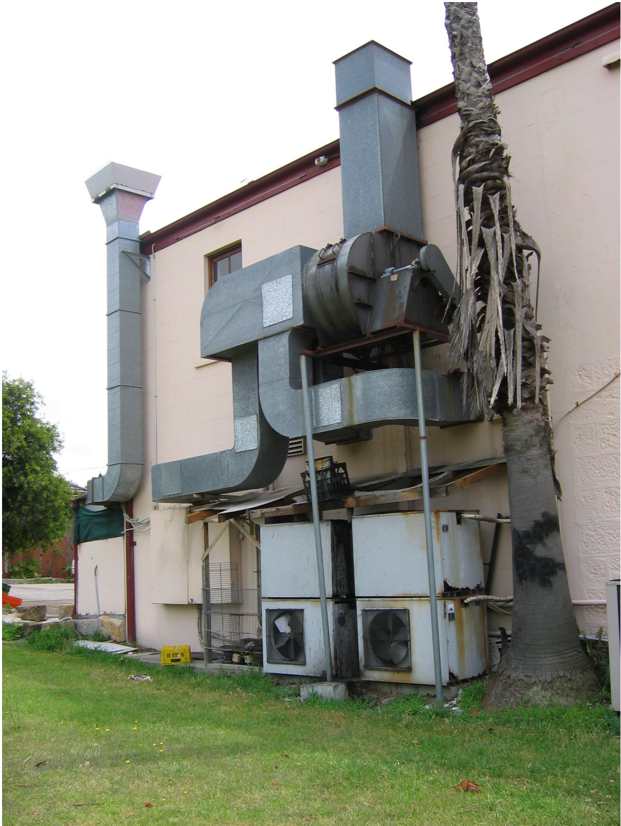
Adjoining private property infrastructure is accessible to park users creating a potential hazard as well as significantly affecting the visual amenity of the parkland.
