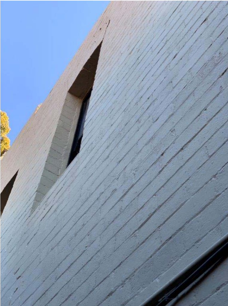
Photo 15 - Cracks in Brick Wall
