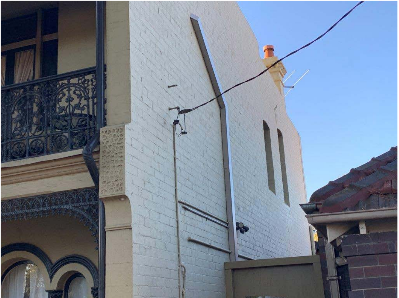
Photo 2 - Cracks in External Brick Wall at Terrace Number 14
