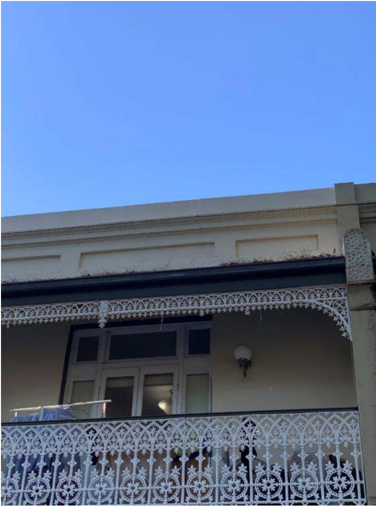
Photo 17 - Cracks in Brick Parapet at Terrace Number 16
