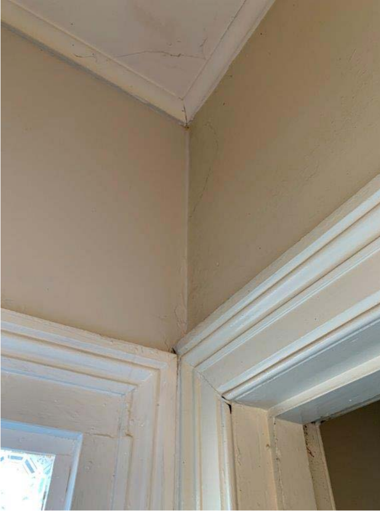
Photo 14 - Cracks in Brick Wall
