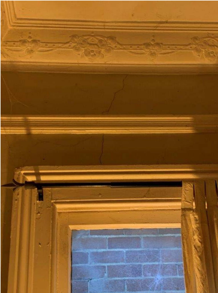
Photo 5 Cracks in Brick Wall
