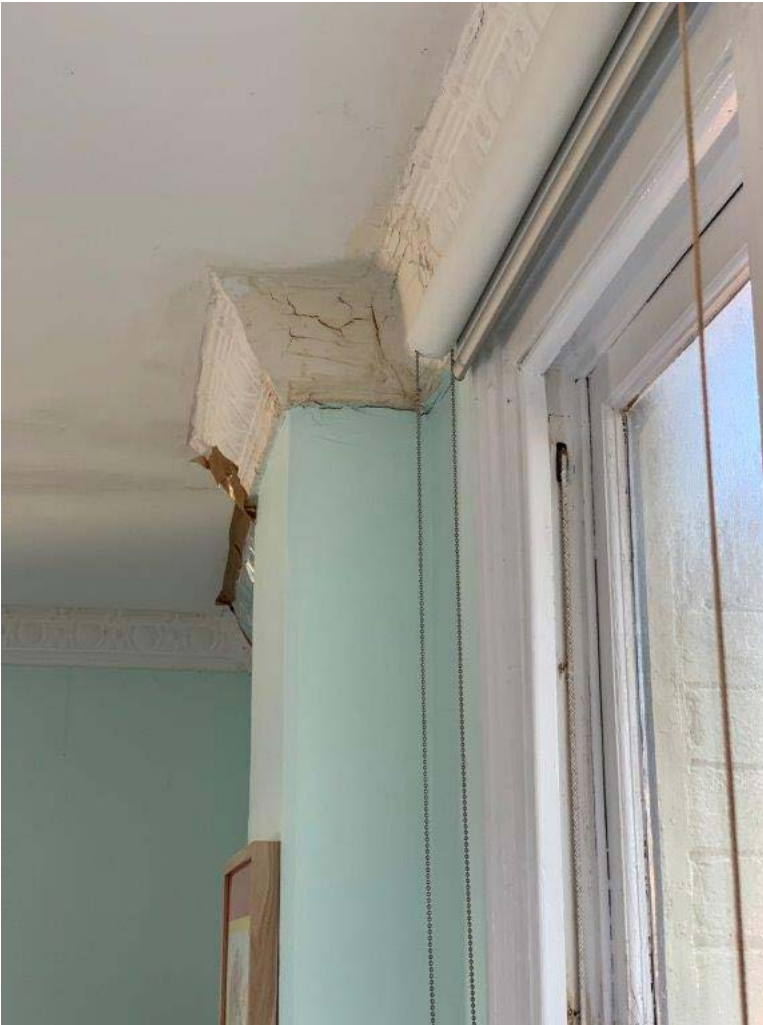
Photo 10 - Cracks in Brick Wall
