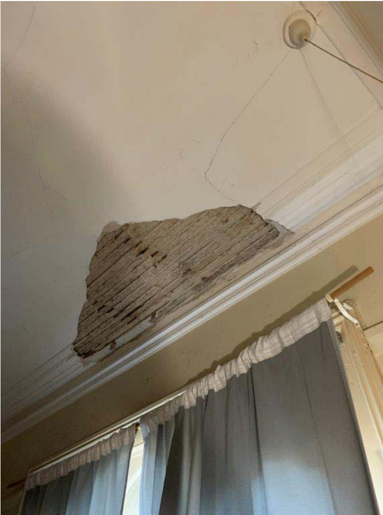
Photo 7 - Cracks in Ceiling and Brick Wall
