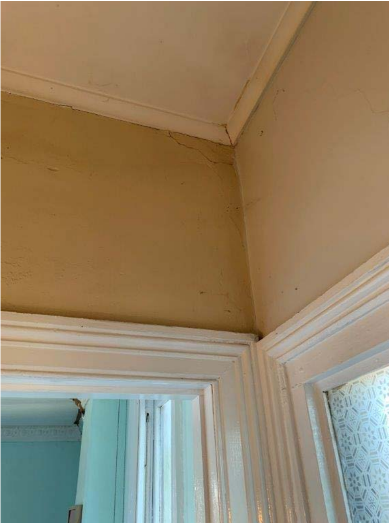
Photo 13 - Cracks in Brick Wall
