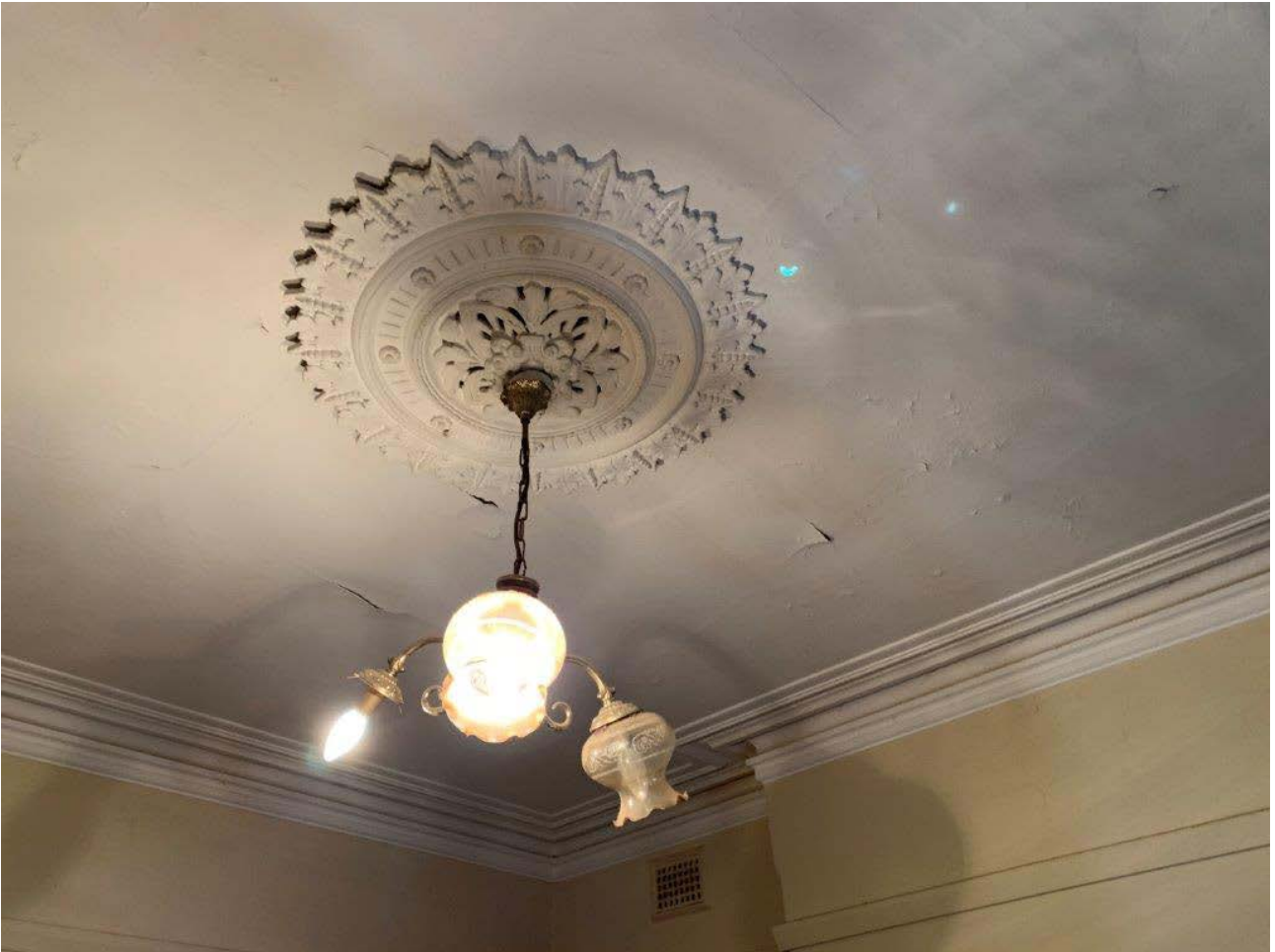
Photo 8 - Condition of Ceiling
