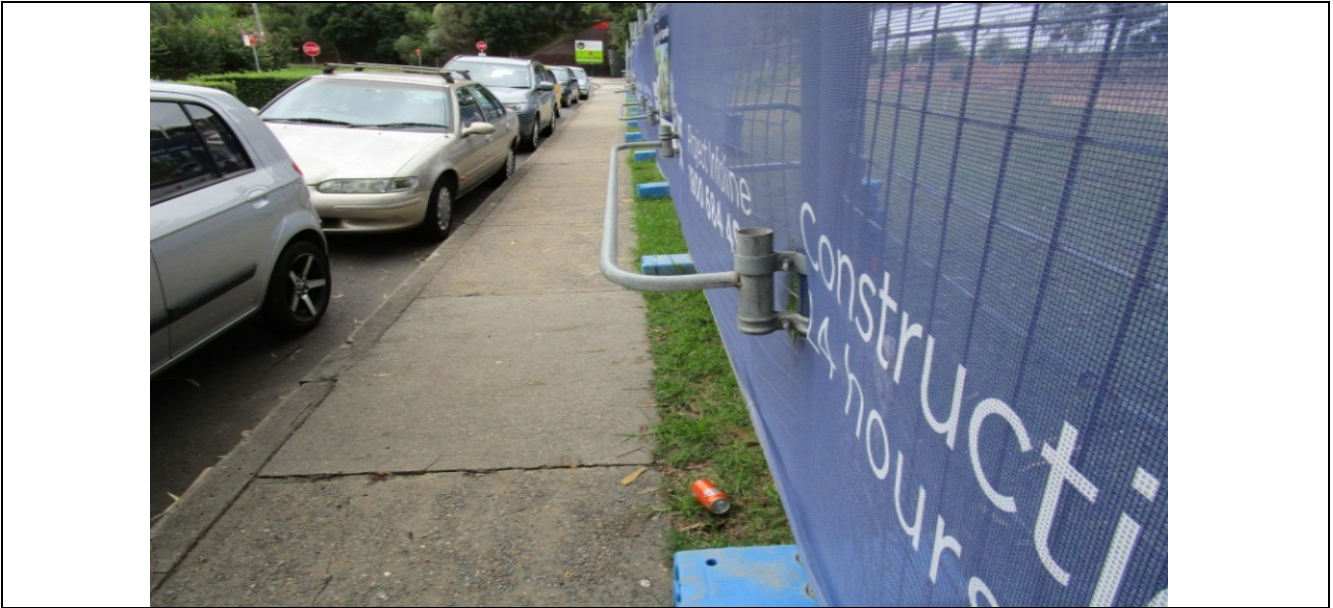
Figure 6: A typical Type C Hoarding fitted with bars to highlight base plates (visual barrier)
