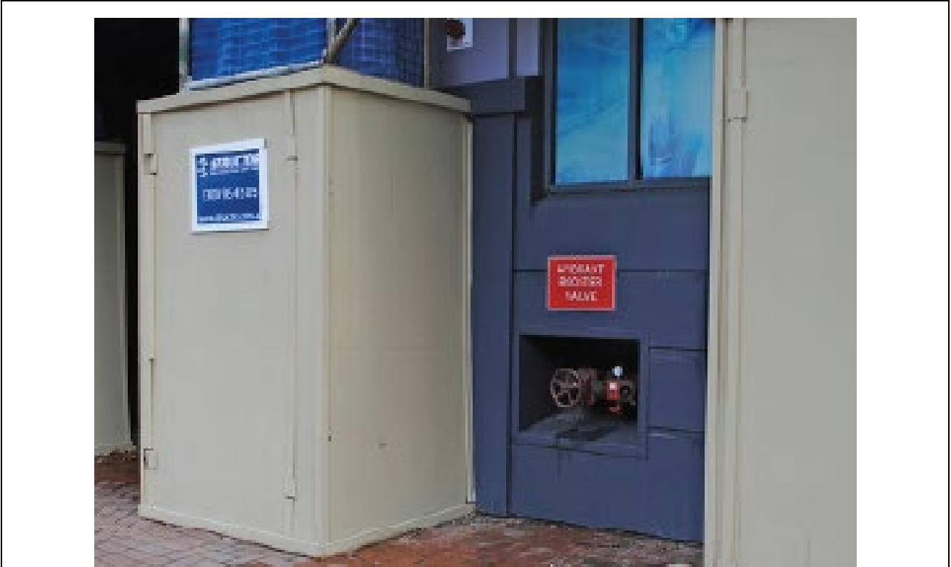
Figure 10: Access to Booster Valve Sets
