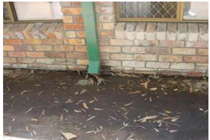
Roof gutters not connected to approved stormwater outlets can cause damage to your property and neighbouring properties
