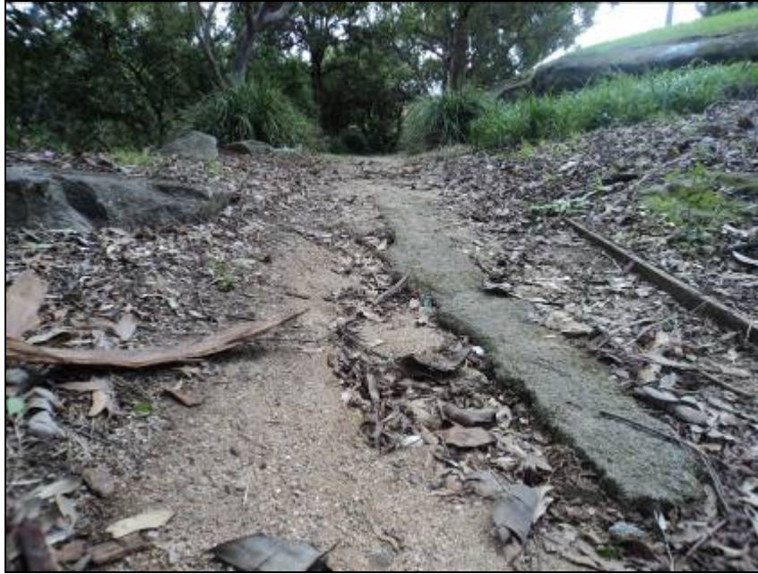
EROSION ON THE MARTIN STREET BUSH TRACK
