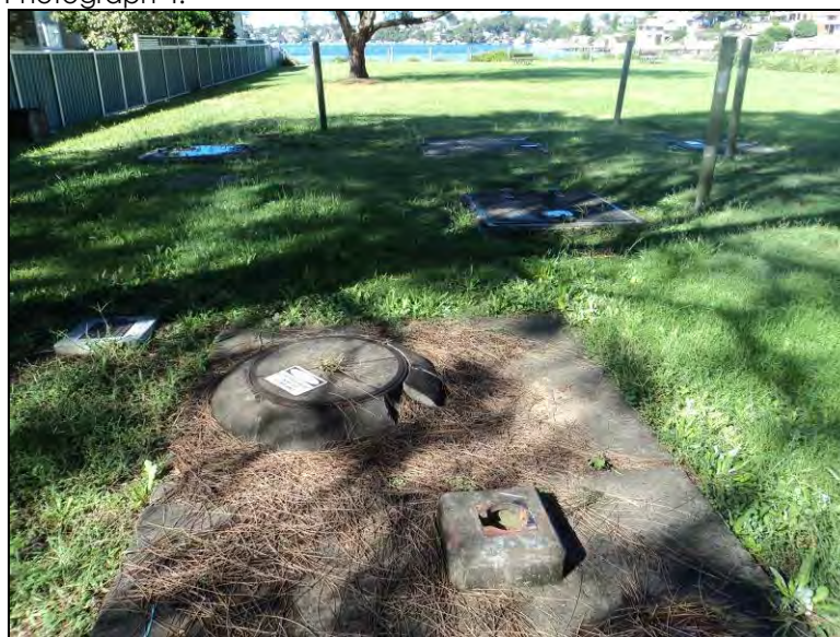
SYDNEY WATER CORPORATION SEWAGE PUMPING STATION SPS 0194
